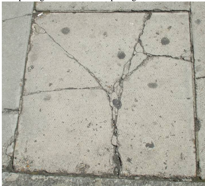
An example of some of the badly damaged concrete paving stones in St James's
